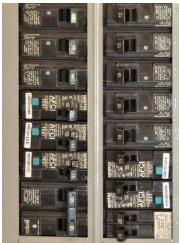
Figure 6. Breaker Box Equipped with GFI Breakers.
